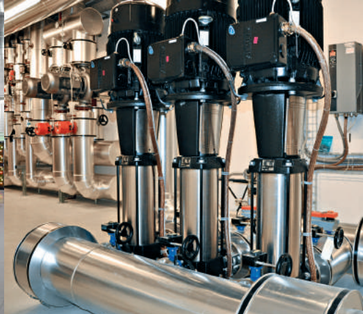
Pumping systems, district heating
